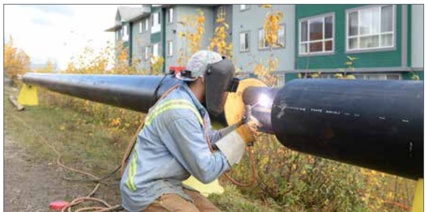
Construction has now wrapped up on the Sustainable Communities Demonstration Project at UNBC.
